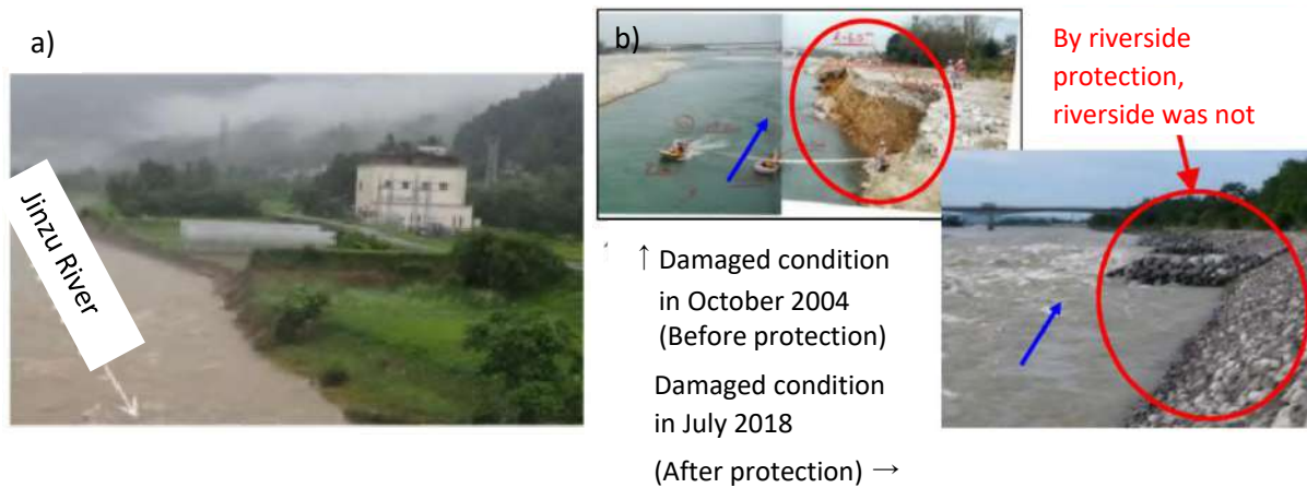
Figure 4: River bank erosion due to flooding and the effect of protection of river banks 3)
